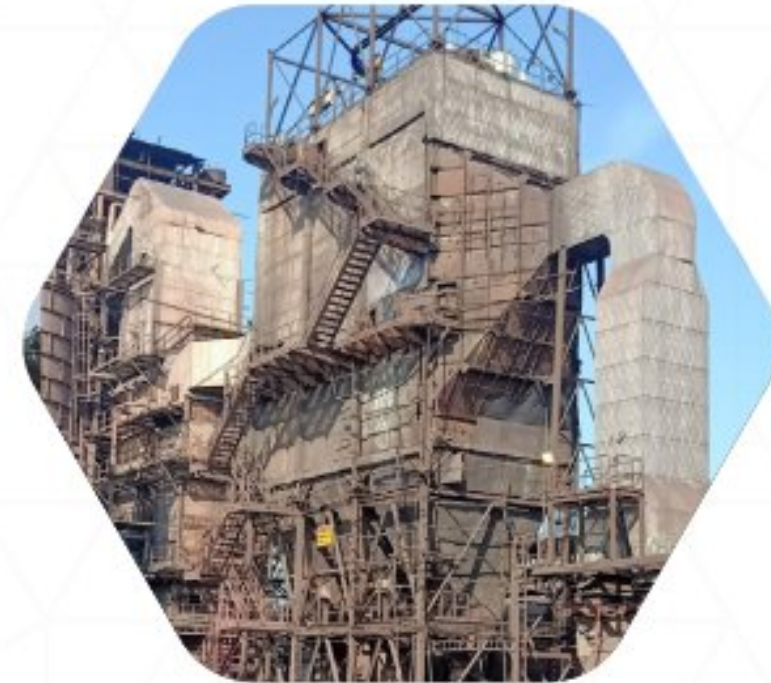
Captive Power Plant Captive power manufacturing
